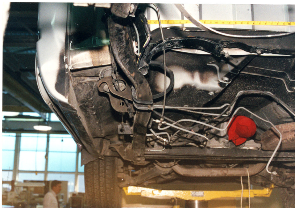
24. View of the left frame rail showing the lateral displacement from underneath the vehicle
